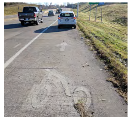
Substandard Bicycle Lane | Shawnee Parkway
