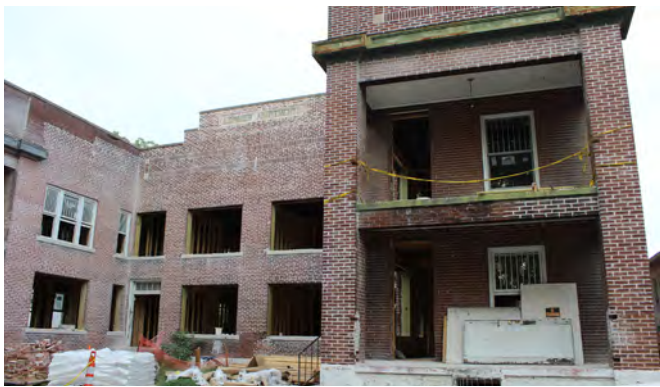
A historic building near downtown is currently being rehabilitated into modern apartments.
