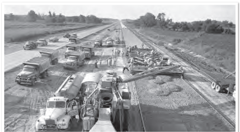
Men and machines near the end of paving of the divided Interstate 55 from Fruitland south to Highway 74 in Cape Girardeau County. This September 18, 1962 photo shows the paving crew, headed south nearing the Bloomfield Road overpass. | Source: Southeast Missourian Archives, G.D. Fronbarger photo
